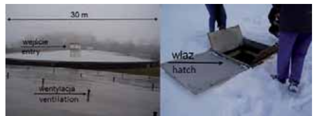
Fig. 2. Tanks for storing water – MPWiK Cracow
